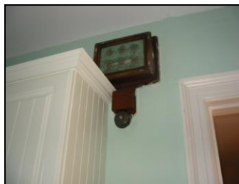
Call bells system in Kitchen
