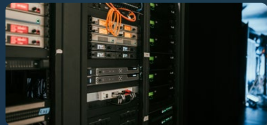
5.95 MVA POWER CAPACITY*
