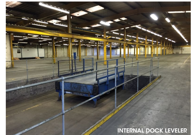
INTERNAL DOCK LEVELER
