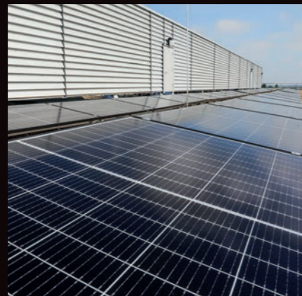
Rooftop solar PV scheduled end of 2022
