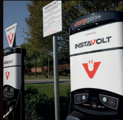
Electric vehicle charging
