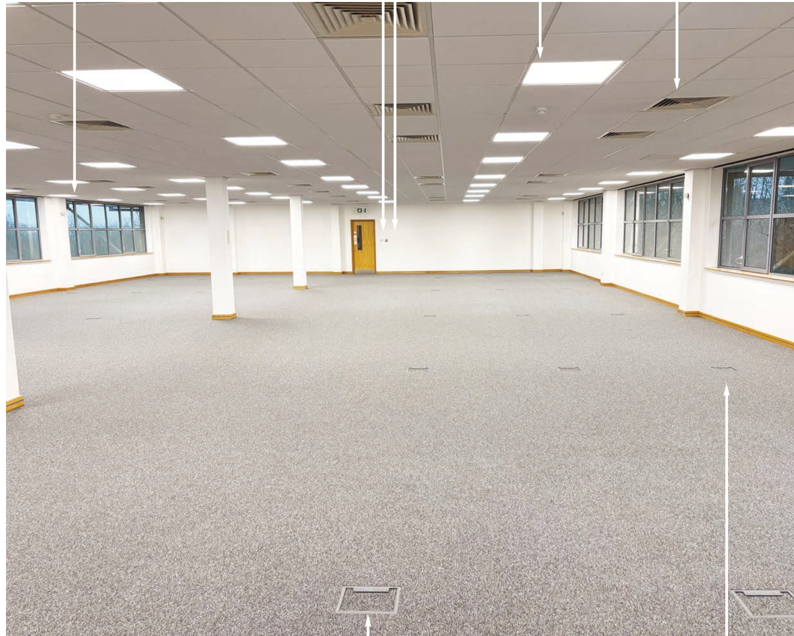
moveable floor boxes in raised access floors with data cabling
