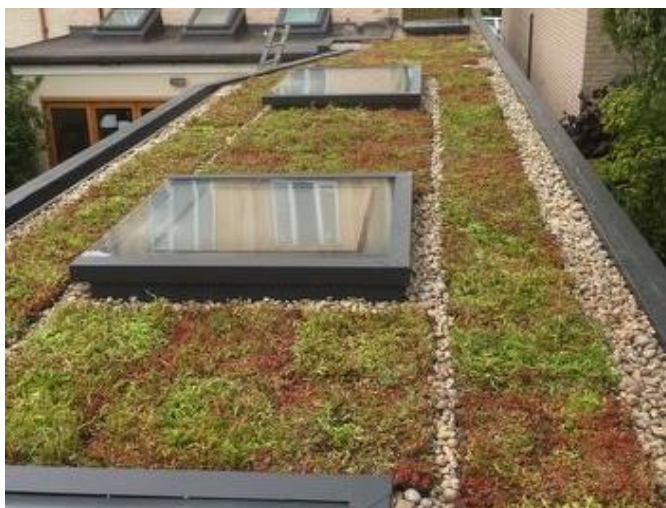
Sedum roof atop the apartment building and above the entrance canopy of the houses
