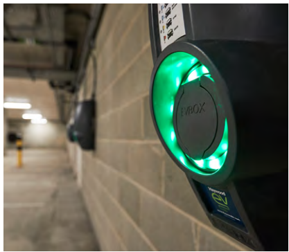
Electric car charging points
