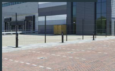
EV car & cycle charging
