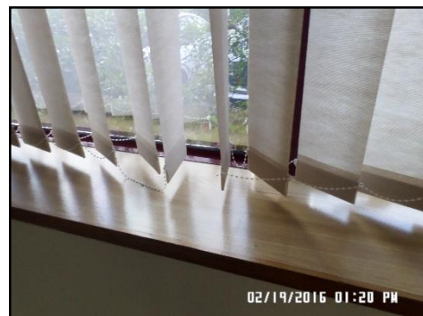
Unusable Area – Window Reveal
