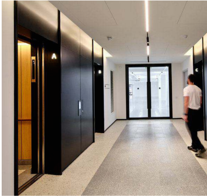
4 x passenger lifts
