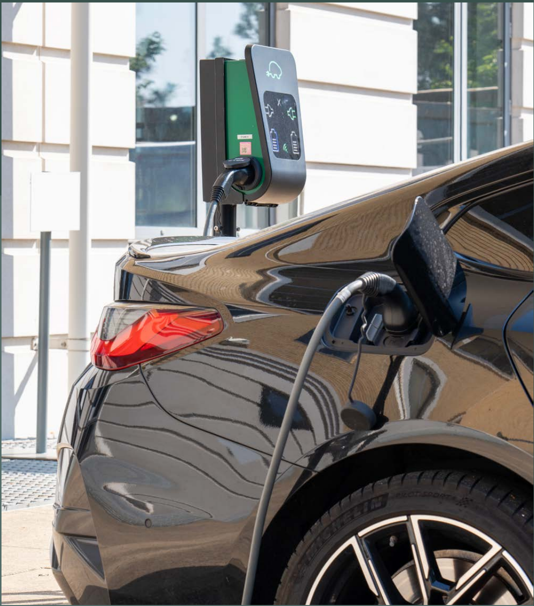
EV charging point
