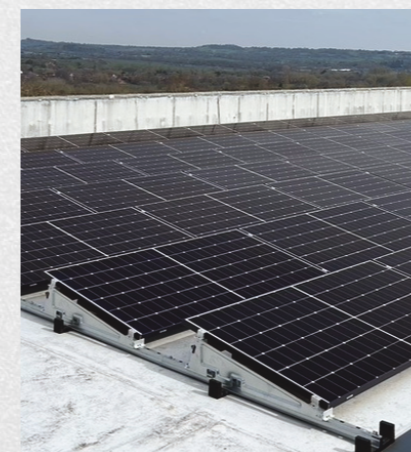
SOLAR PANELS ON ROOF
