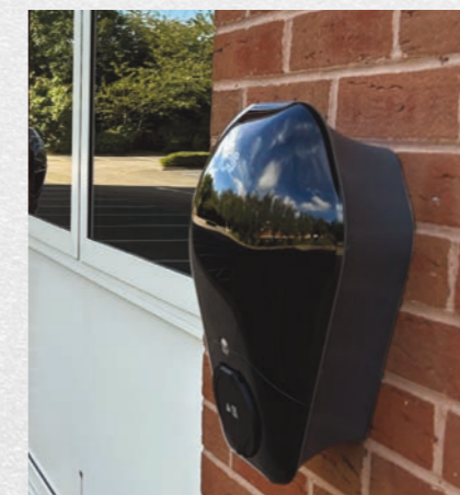
7kW EV chargers
