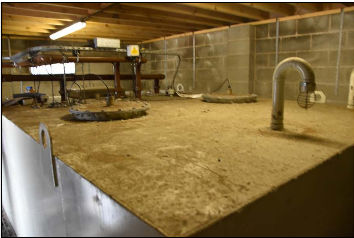
Plate 6 Tank-no olfactory odours
