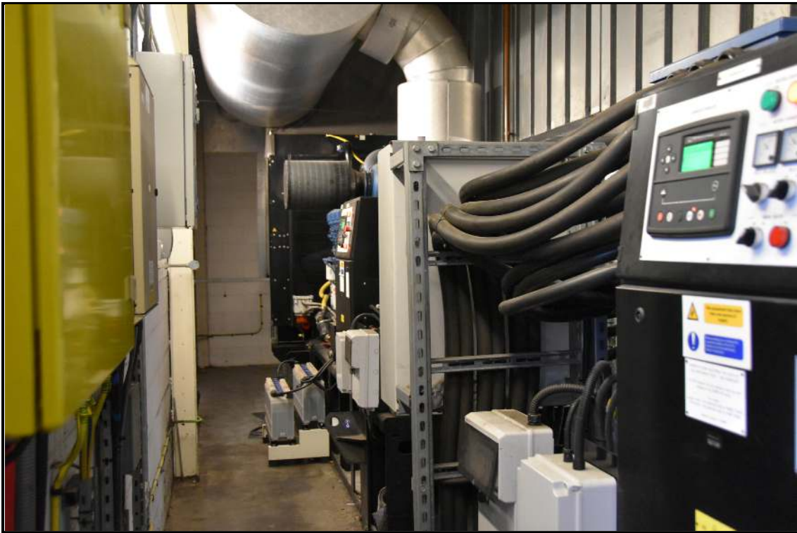
Plate 7 Generators with day tanks
