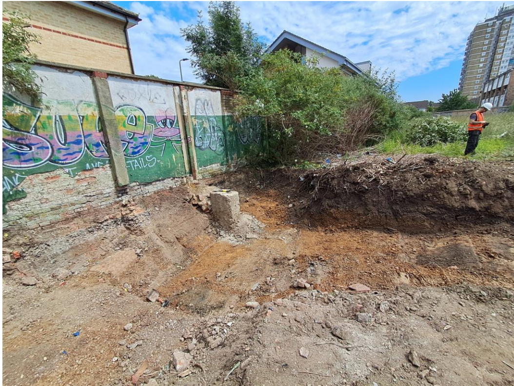
Excavations carried out near the boundary wall. We found JKW rhizome growing into and underneath the wall.
