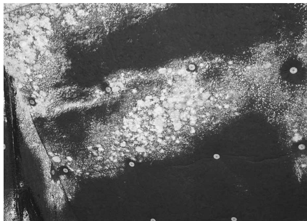
Fig. 3 Fungal colonization of the lining of an air-handling unit in a building. Culturable Aspergillus fumigatus was recovered from this area. The supply airstream passes directly over this surface, which is often located after (downstream) the filters.
