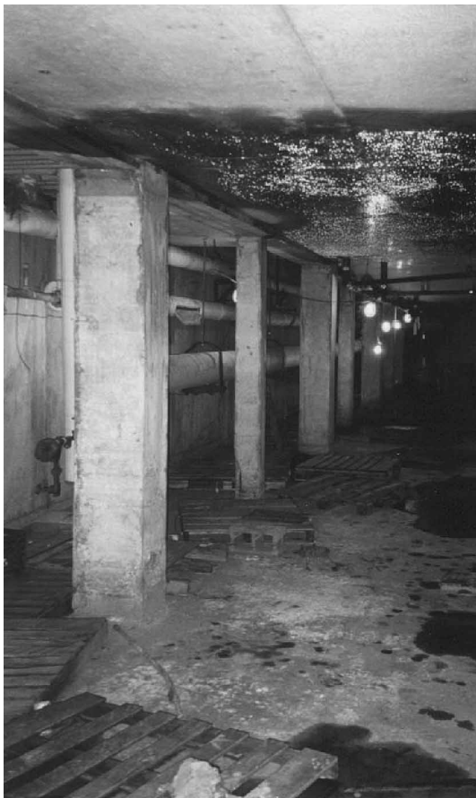
Fig. 2 Tunnel through which outdoor air is routed into the ventilation system of a building. Note water that has collected in the tunnel and wooden pallets and other debris that are wet and in the airstream passing through the tunnel.
