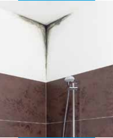
Wall affected by mould
