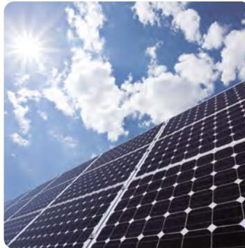
Photovoltaic energy generation at EVVA
