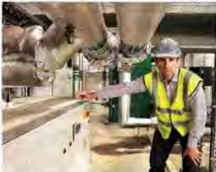
WARMED UP James Howard director of the Lakeshore development, with the ground source heat pump
