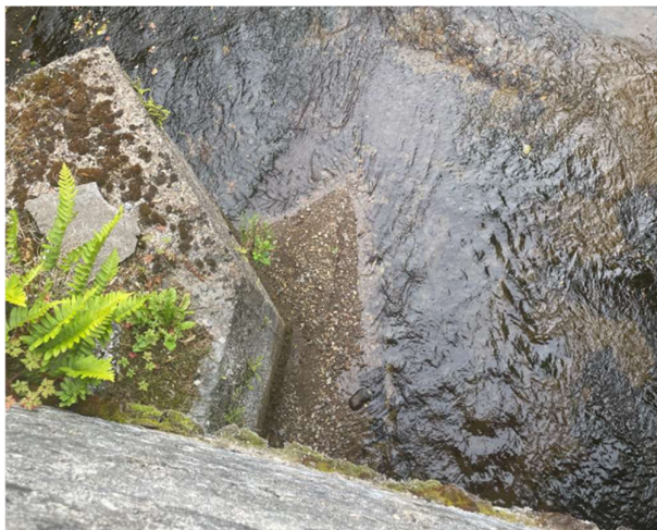
Figure 4-52 Base of bridge is visible and gravel sediment deposited around pier.
