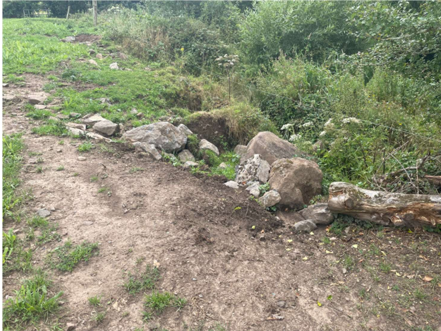
Figure 4-21 Right bank failing and slumping into the river. Additionally exposed fine sediment which could contribute to sediment load during local runoff event.
