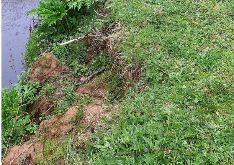
Figure 5-4 Bank Slippage happening on River Slievenohera.
