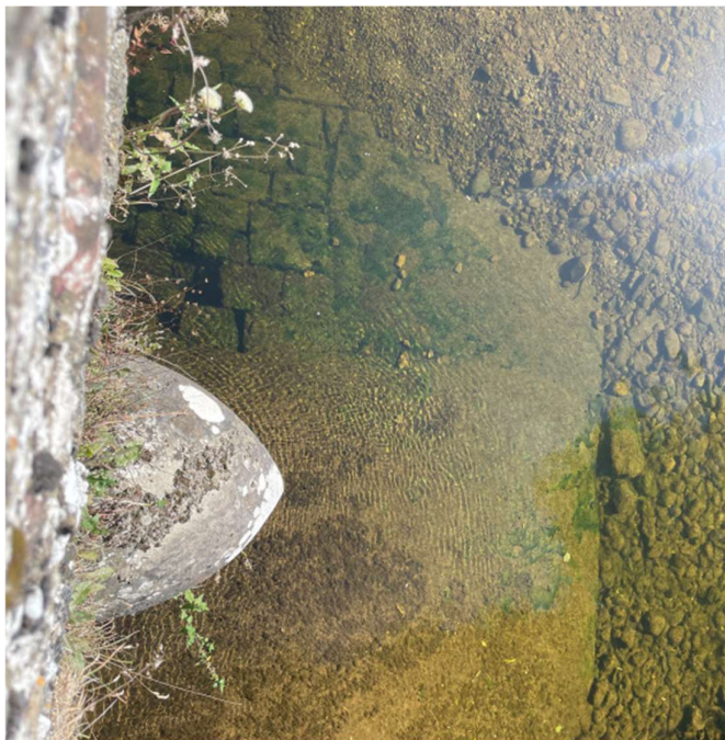
Figure 4-35 Coarse bed material scoured from bridge upstream from weir structure (structure not undermined).
