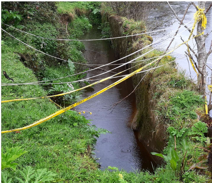
Figure 5-5 River Slievenohera has eroded behind failed timber ramps.
