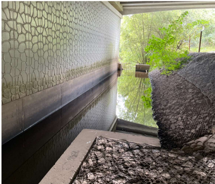
Figure 4-7 Scattered flood trash (leaves/reeds etc.) evident up to the bankfull location on the rip-rap (left bank).
