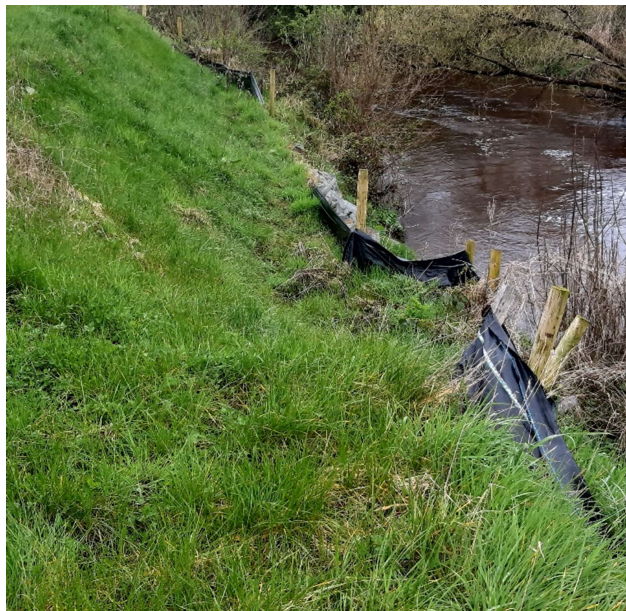
Figure 5-3 Bankside fencing/protection which is slipping into the River Newport.
