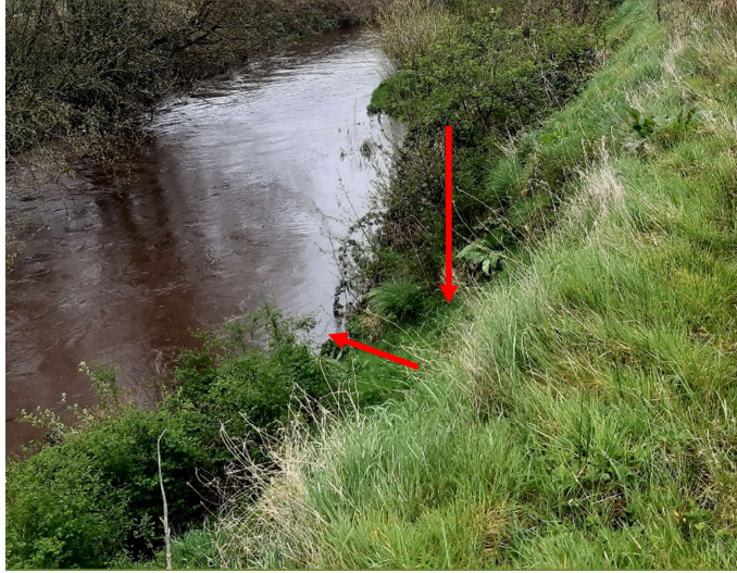
Figure 5-2 Bank slippages along the River Newport.
