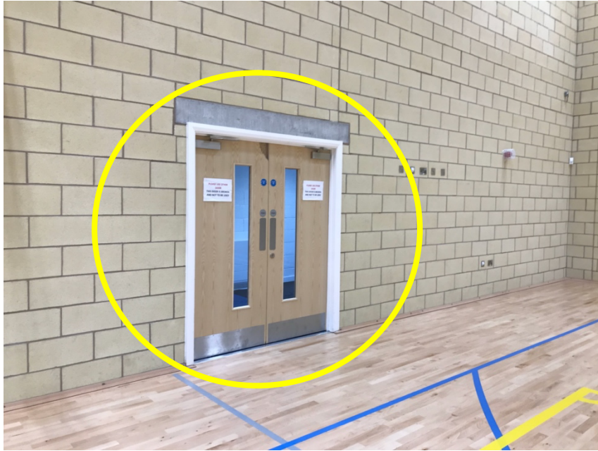
One-way exit route out of the Sports Hall into the one-way corridor (above)
