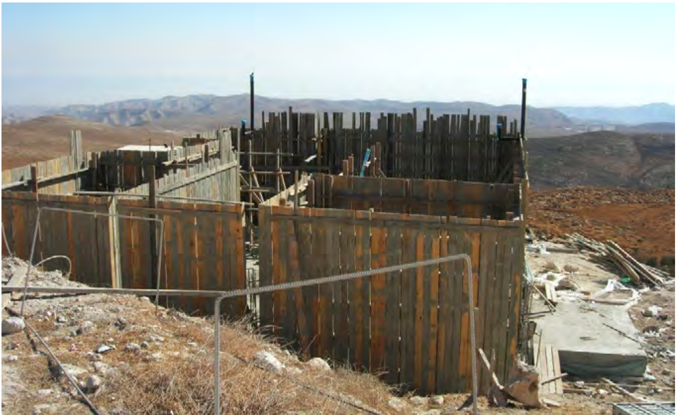
Construction in the outpost of Mitzpeh Danny, October 2010. Established on public land in Deir Dobwan Photo by Yesh Din
