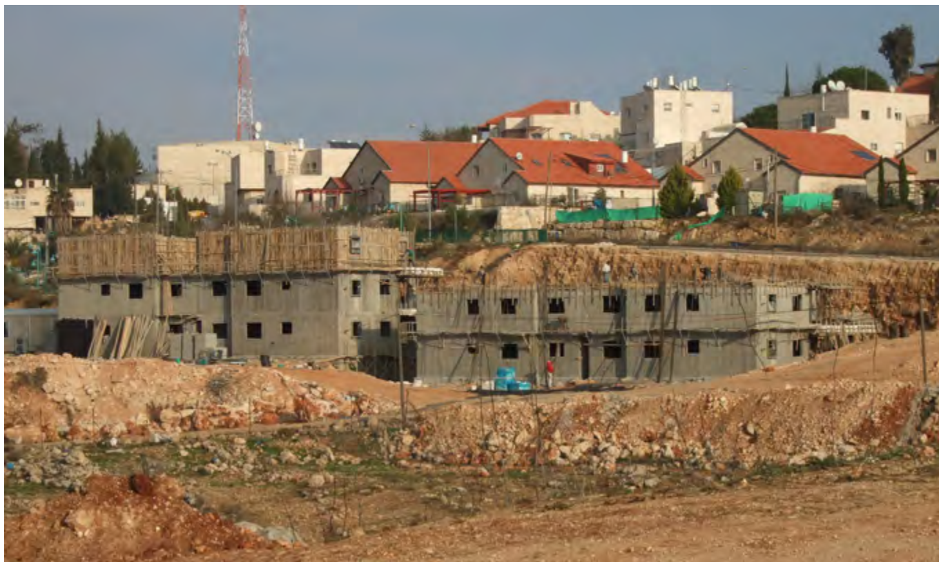
Dura al-Qar', January 2011. While the land was seized for military needs, two residential buildings were established on it in the settlement of Beit El Photo by Yesh Din
