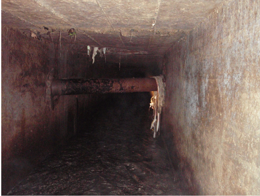
Figure 2-1 Obstruction in Wad Culvert
