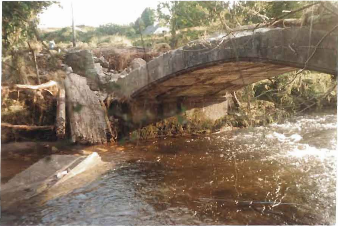
DESTRUCTION OF PŪL NA BRŌ BRIDGE PHOTOGRAPH NO. 1
