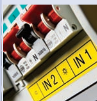
Distribution boxes & patch panels
