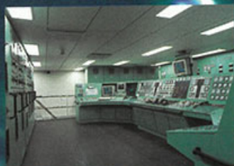
Engine control room console
