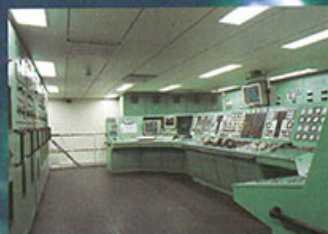
Engine control room console
