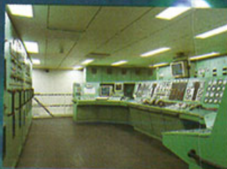
Engine control room console
