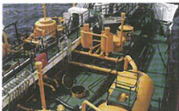
View of oil-water separator
