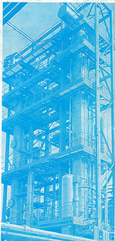
Two-column continuous rectifying plant built by Sulzer in Switzerland.
