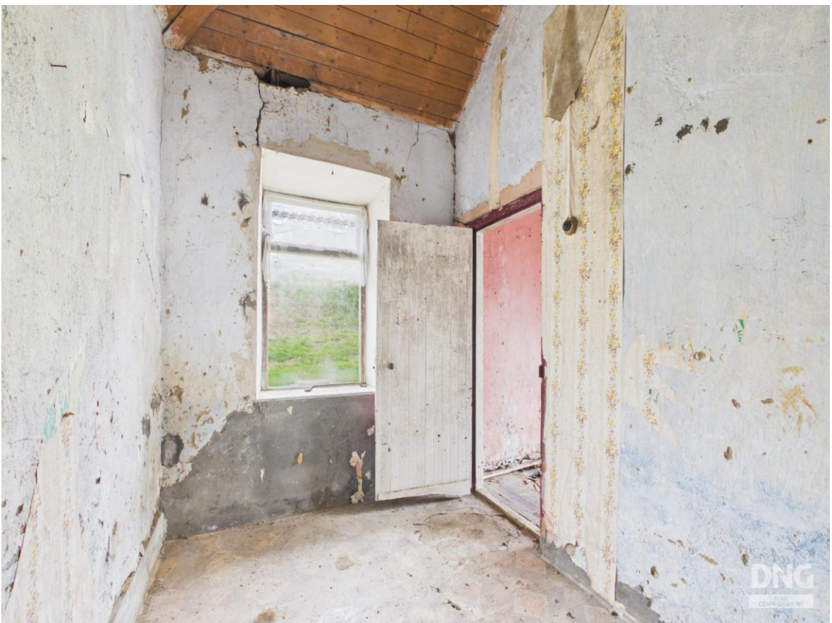
Derelict Residence, Ashbrook, Strokestown, Co. Roscommon
