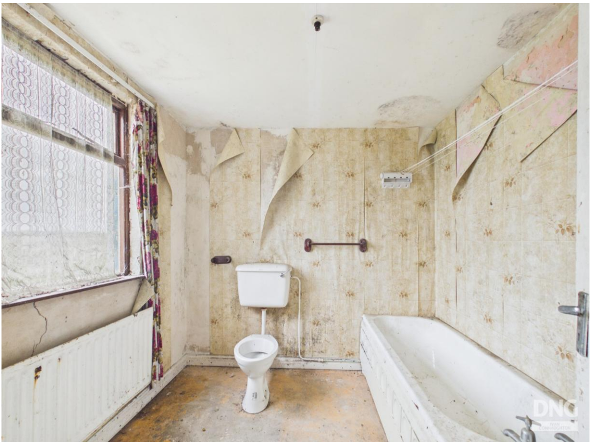
Derelict Residence, Ashbrook, Strokestown, Co. Roscommon
