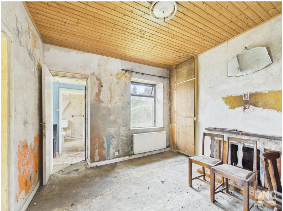
Derelict Residence, Ashbrook, Strokestown, Co. Roscommon
