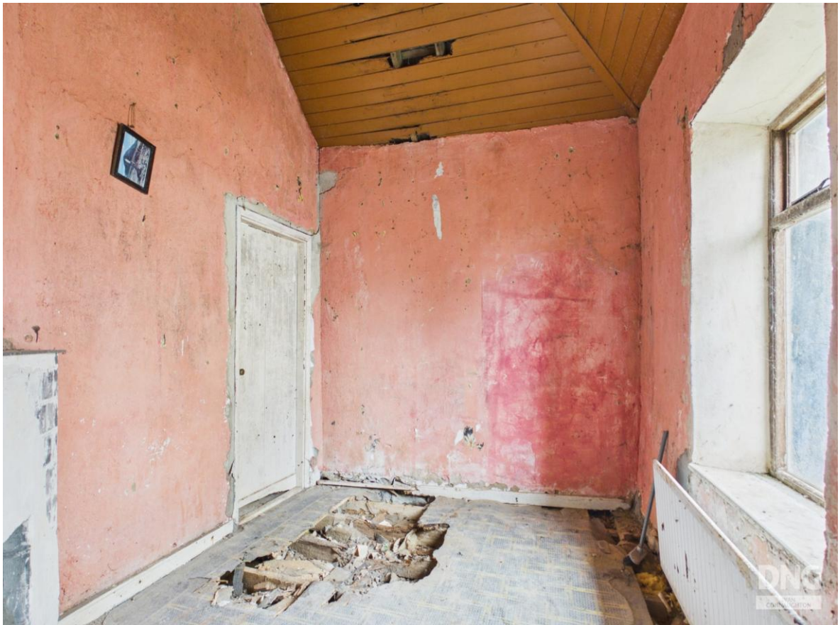
Derelict Residence, Ashbrook, Strokestown, Co. Roscommon
