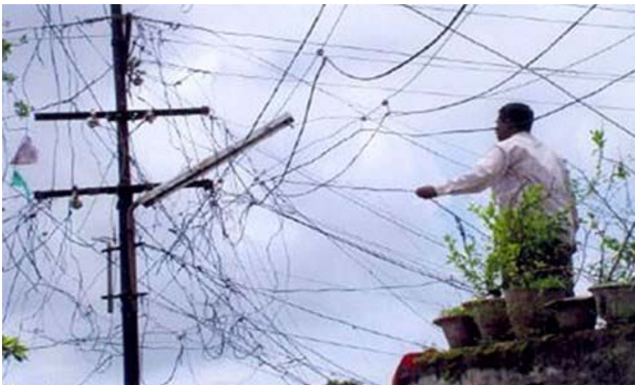
Figure 6: Tapping electricity directly from a distribution feeder - bypassing the meter.
