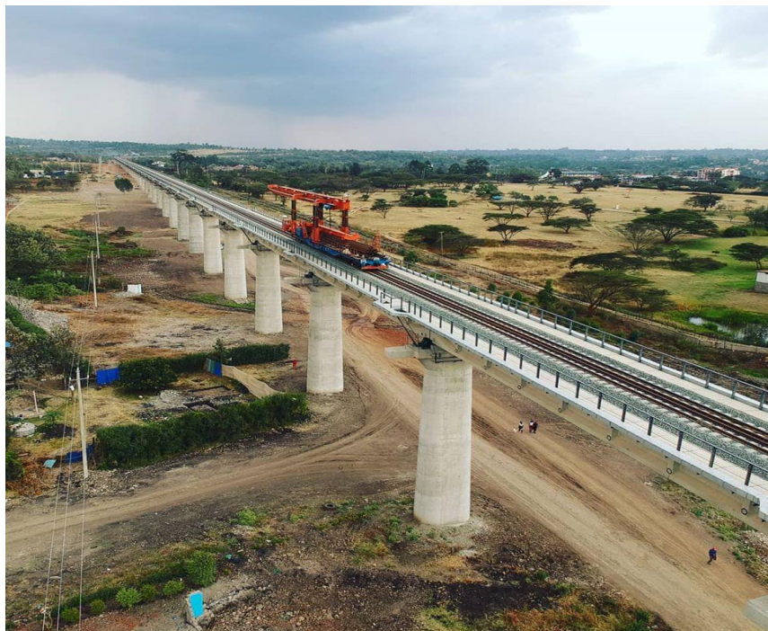
Figure 4 A section of the on-going construction of the Standard Gauge Railway (SGR), This is a flagship Government of Kenya project in collaboration with the central government of the People's Republic of China, photo provided with permission to share from Moonlight Media Services, Aug 31, 2019
