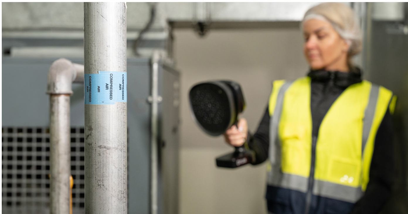
Acoustic imaging camera helps maintain top performance by identifying small leaks in critical compressed air systems.
