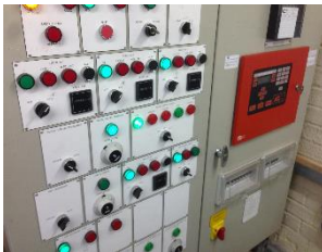
Boiler house 1. Key: 42 Location: KS1 playground
