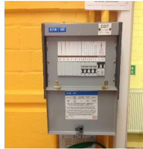
Electricity Fuse Box Location: Intervention Room
