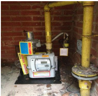
Gas Outside Reception area Key: 50 Turn lever on left hand side to switch off
