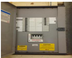
Electricity Fuse box Location: Room of Imagination on wall at the back Switch off the 4 switches in the middle
