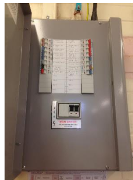
Electricity Fuse Box Location: Year 6 Switch off the switches in the middle
