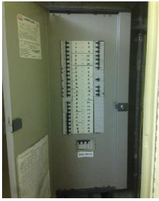
Electricity Fuse Box Location: Hall
