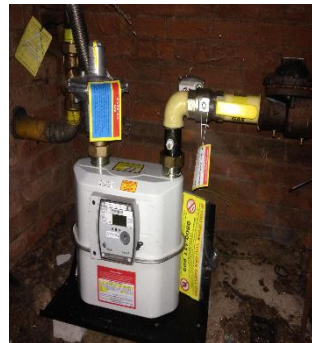
Gas Location: Outside the main entrance Key: no key needed Turn lever on right hand side
