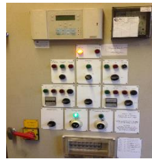
Boiler house 2 Key: 42 Location: Reception area
