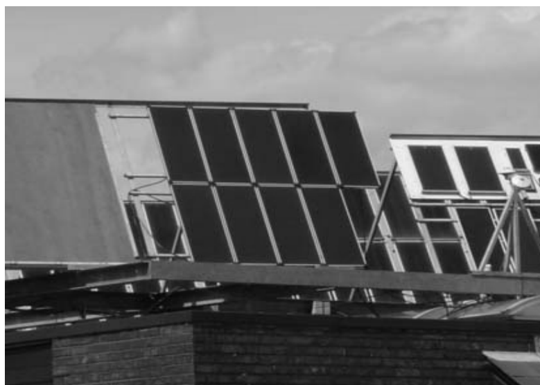
Figure 1: Nine a-Si modules with 4 different i-layer thicknesses were installed in the outdoor measurement system on the CREST building
