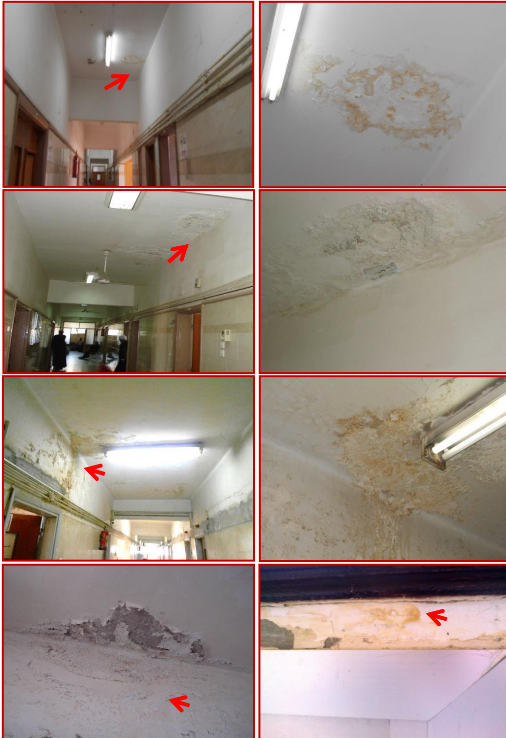
Photos of deteriorated paint samples collected from different sites in Assiut University hospitals.
