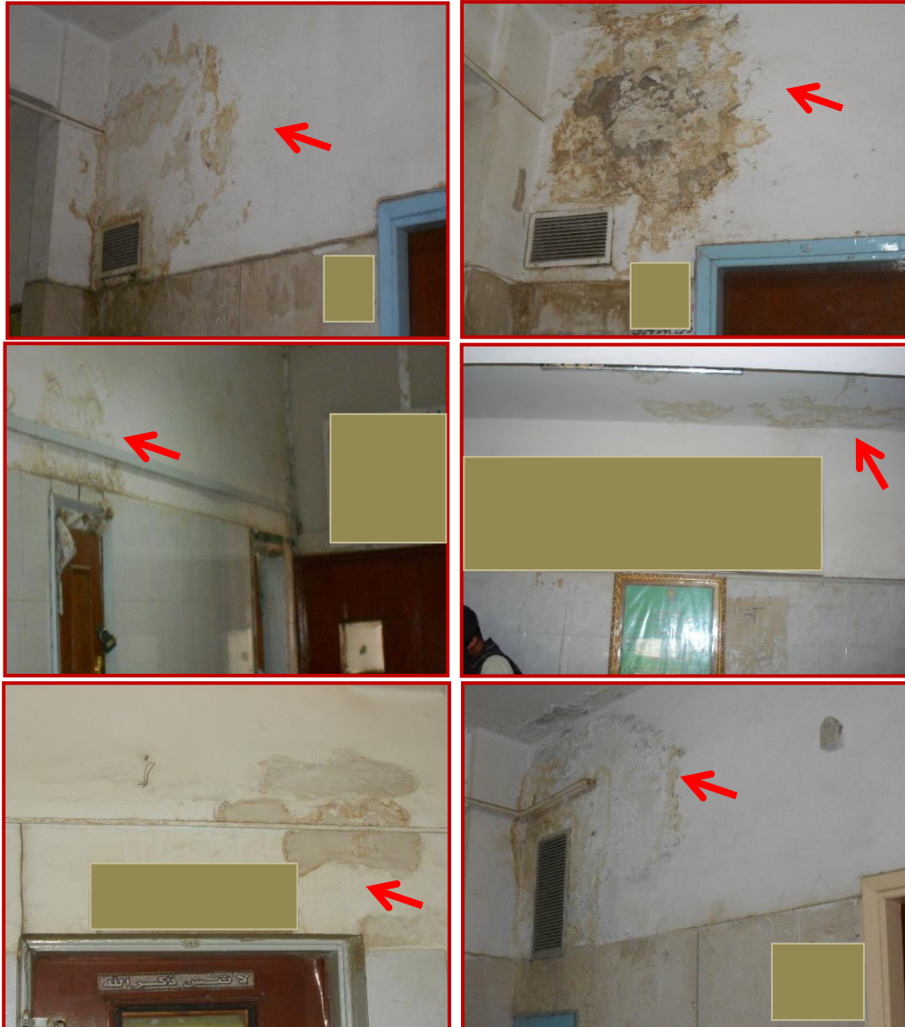
Photos of deteriorated paint samples collected from different sites in Assiut University hospitals.
