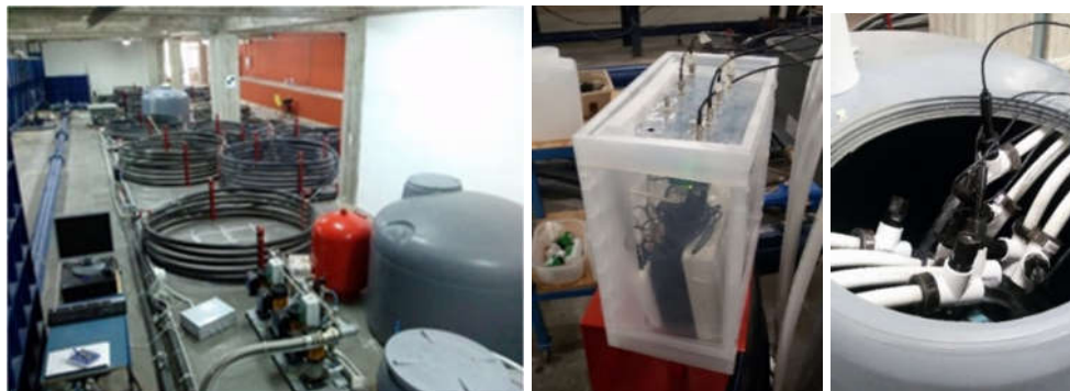
Figure 2. Overview of the water distribution network and placement of conductivity sensors.
