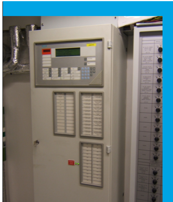
Typical automatic fire alarm panel
