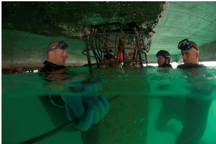
U.S. Army Engineer divers building a rebar cage for a pile cap.
