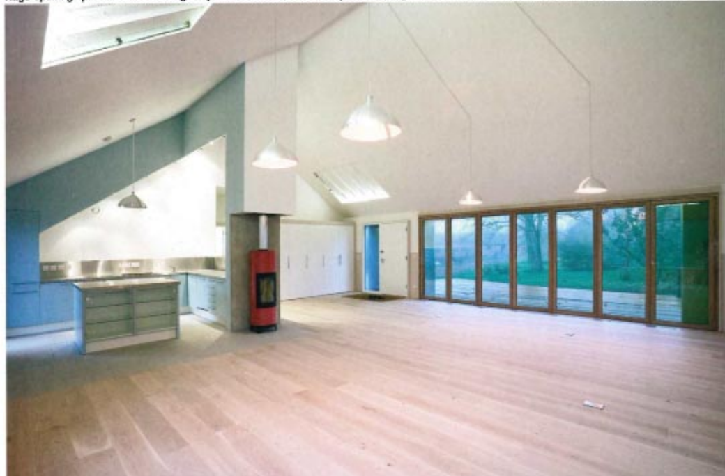
Two ceiling panels have been left off in the living/kitchen area, above the door and diagonally opposite, to reveal the panel system beneath.
