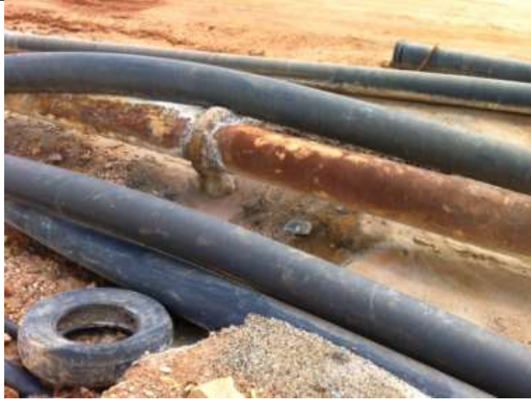
Poor management and maintenance of pipeline infrastructure
