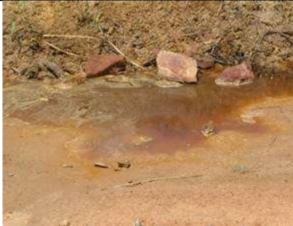
Polluted water seeping from Lancaster Dam wall into the Upper Wonderfonteinspruit
