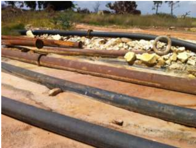
Poor maintenance and management of pipeline infrastructure.
