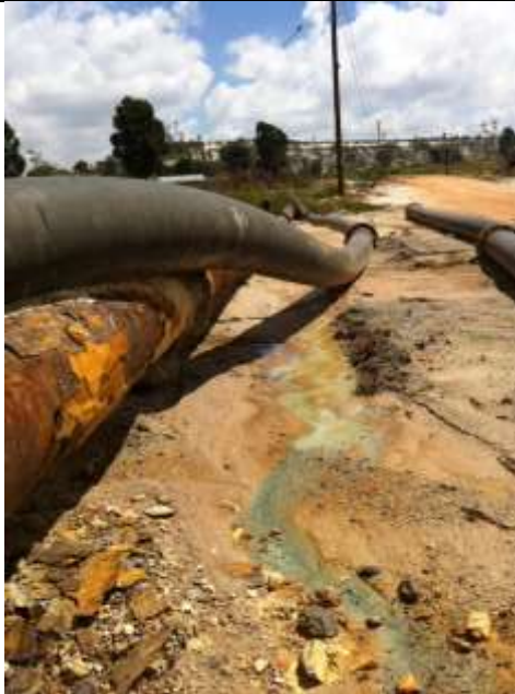
Poor management and maintenance of pipeline infrastructure, and regular spillages adjacent to a wetlands.
