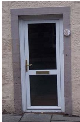
Poor door replacement
