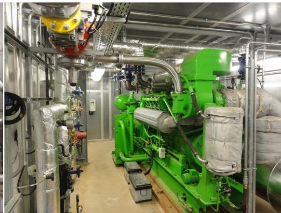
Figure 3 – 500 kW CHP unit
