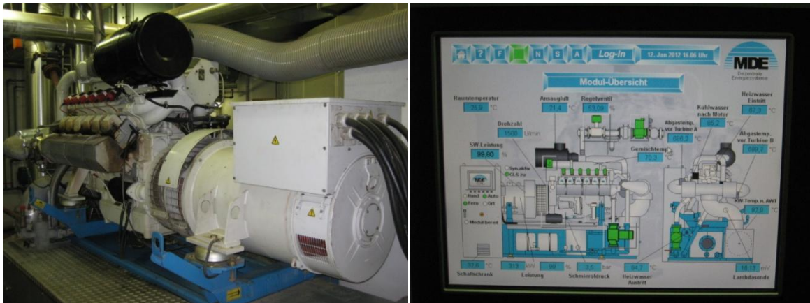
Picture 1: MDE biogas engine with control panel
